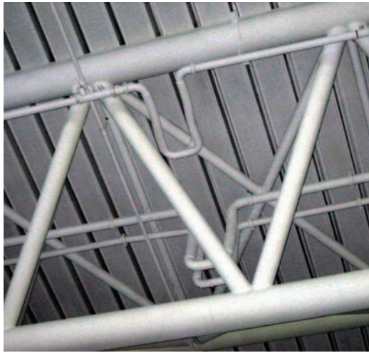
Fireloops designed for 12-inches of movement were installed in the ceiling to allow for roofs movements of up to 5-inches upward and 1-inch downward.
